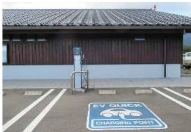
Yakushima Town Hall Standard Charging Station (1 unit)
